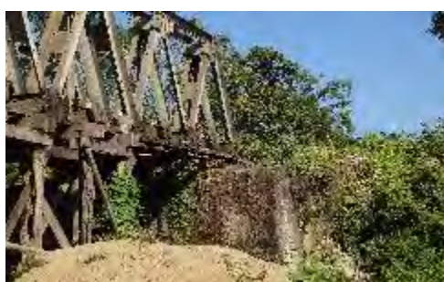
(Deformed abutment and wooden piers)
