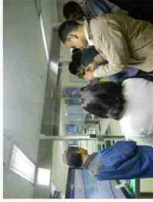
Control room (SCADA)
