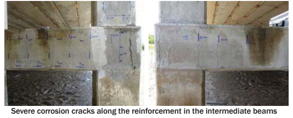
Severe corrosion cracks along the reinforcement in the intermediate beams
