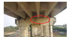
Crack in neighboring pier
