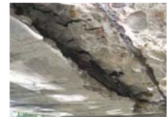
Significant corrosion of main rebars
