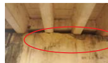
Crack under anchorage
