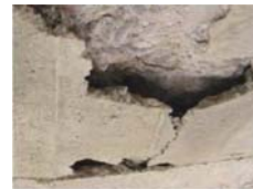
Delamination of concrete
