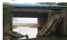
After the bridge fell down
