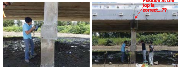
Strange shape observed in the columns
