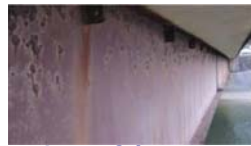
- State of the outer surface of the girder -
