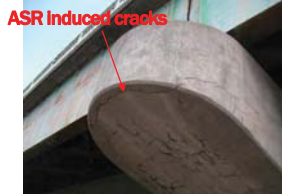
Damage by ASR (Alkali Silica Reaction)
