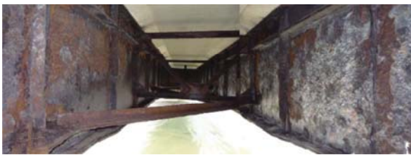
-Corrosion state of the girder inner surface-
