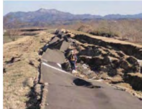
River Dike Collapse
