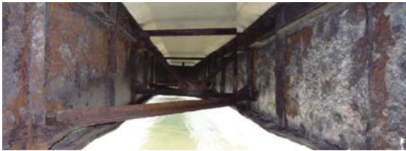
-Corrosion state of the girder inner surface-
