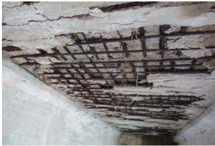
Severe corrosion of steel reinforcement in slabs (already replaced to new one) The girders just besides the slabs are sound. See water or sand was used for the slabs?
