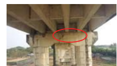
Crack in neighboring pier
