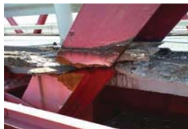
Breakage of diagonal Member in truss bridge
