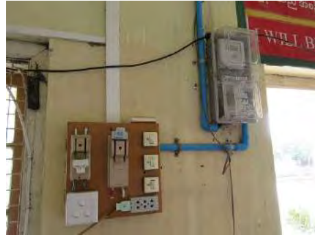
Figure 5.9.11 Lighting system of platform Figure 5.9.12 Electric power system and socket outlet system
