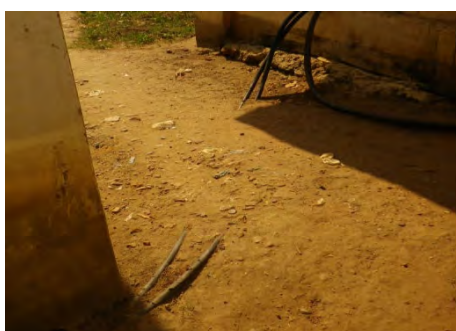
Figure (a) OFC (underground)
