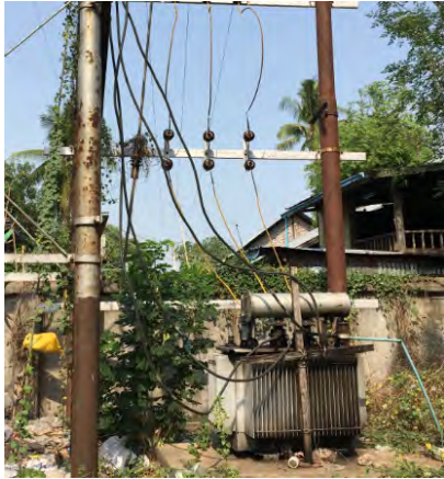
(a) High Voltage Receiving Equipment in a Station
