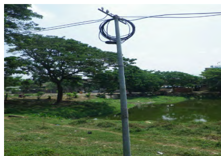
Figure (b) OFC (Overhead Line)
