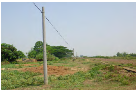
Figure (a) OFC (Overhead Line)
