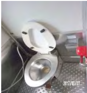
(c) Western-style Toilet
