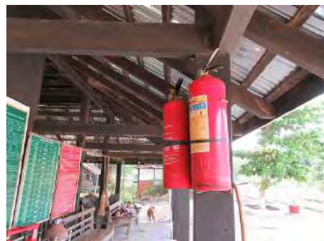
Figure 5.9.14 Fire extinguishing facility
