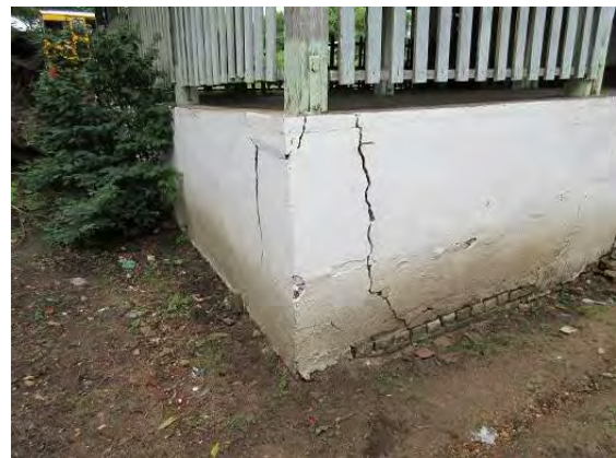
Figure 5.9.4 Crack of foundation
