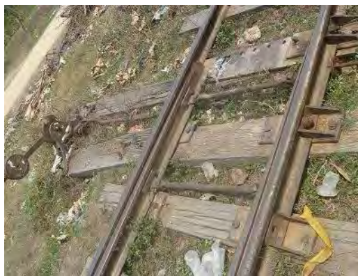
(c) Turnout and Point Machine without Proper Maintenance
