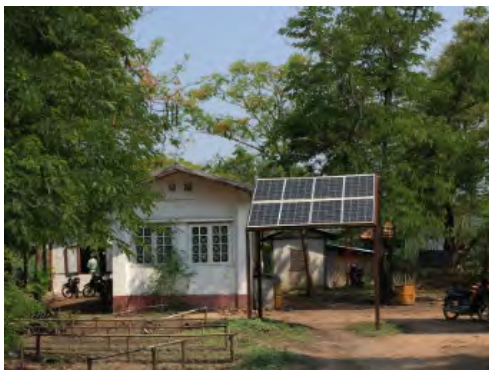
(e) Solar Power System
