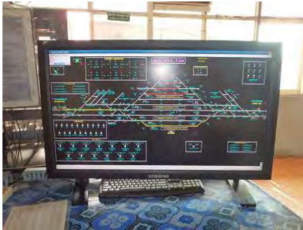
(a) Interlocking Control panel
