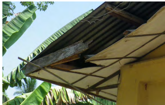
Figure (b) Damage of Roof
