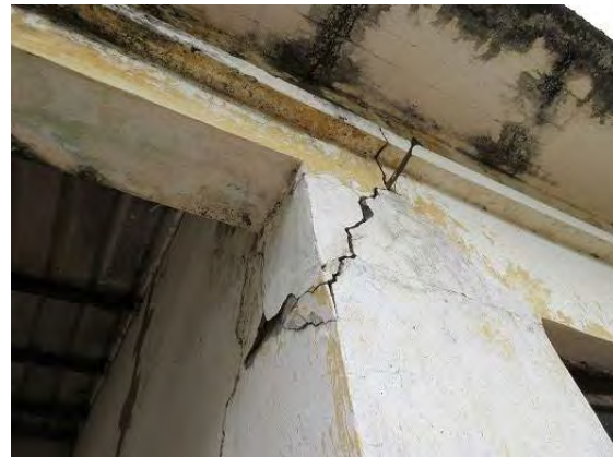
Figure 5.9.8 Crack of Ingyinkan Station
