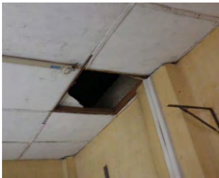
Figure (a) Hole of Ceiling
