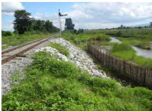
(c) Settlement due to erosion by stream (Mile 243)
