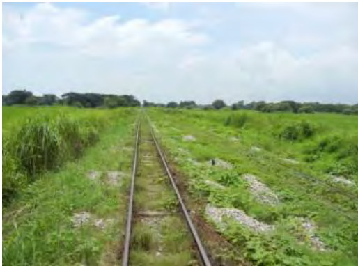
(a) Settlement due to soft ground (Mile 82)
