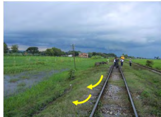
(b) Settlement due to soft ground (Mile 146)
