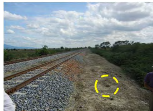
(d) Settlement due to unstable embankment (Mile 336)
