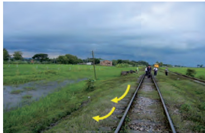
Photo.4 Settlement due to soft ground (Mile 146)
