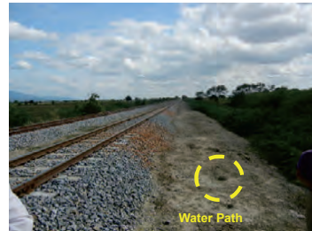
Photo.6 Settlement due to unstable embankment (Mile 336)
