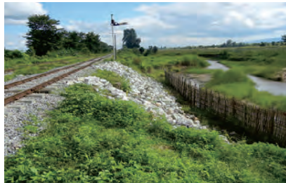
Photo.5 Settlement due to erosion by stream (Mile 243)
