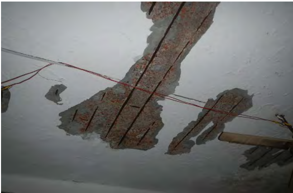
Roof slab steel bar rusted, Hazaribag GOD
