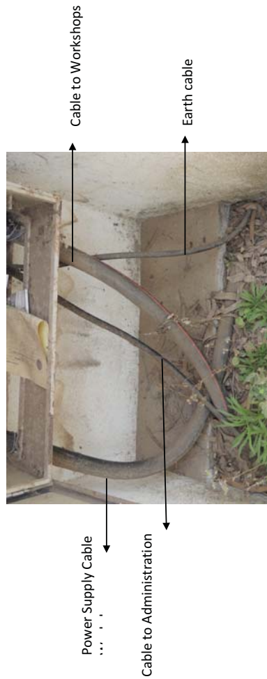
Figure 27. Cables at the Transformer
