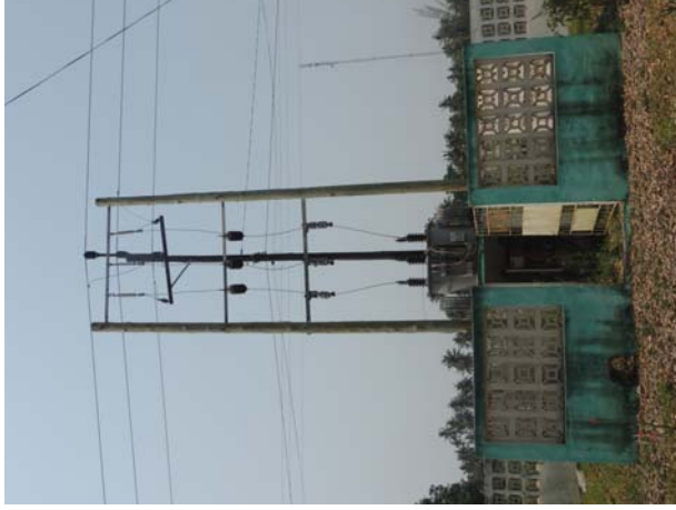
Figure 24. General view of Transformer
