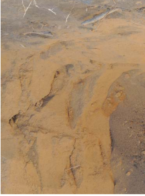
Figure 19. Detail of internal erosion
