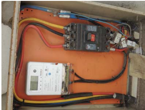
Figure 26. Main switch at Transformer
