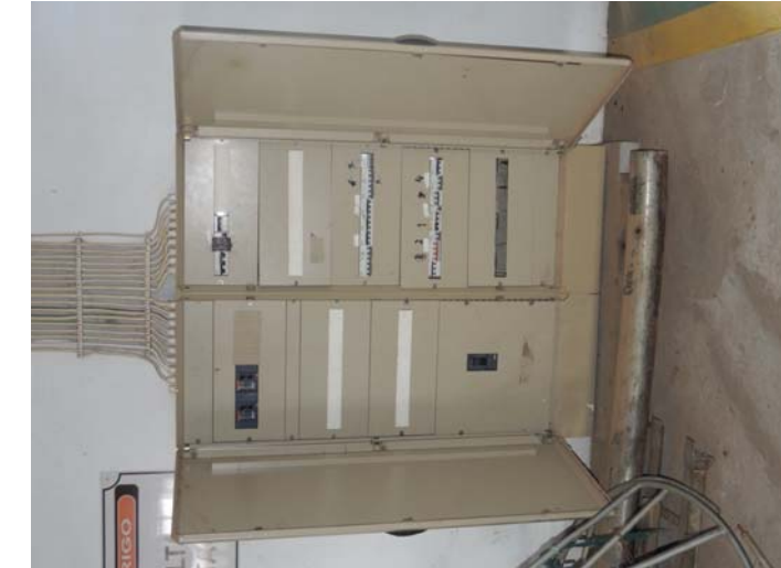
Figure 18. Main Distribution Board, in the Joinery workshop
