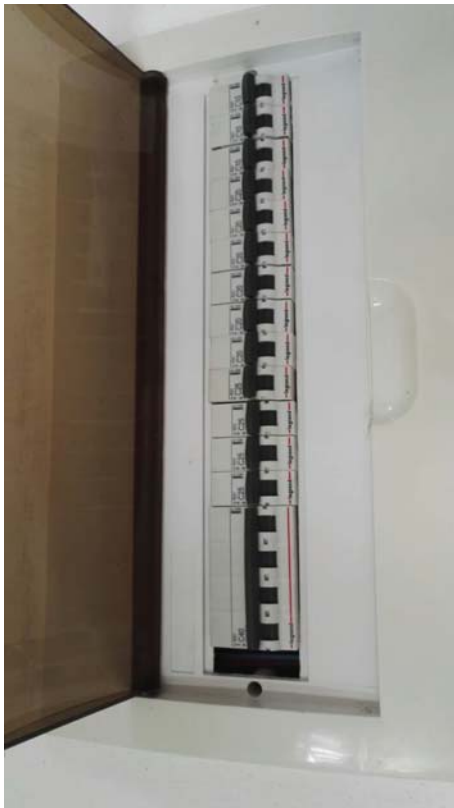
Figure 22. EB at the Administration Building
