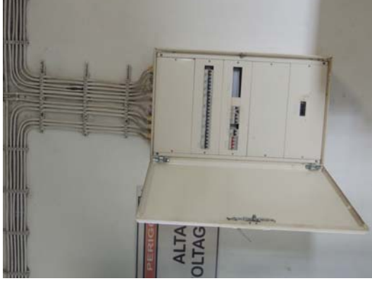
Figure 20. Control board of locksmith workshop
