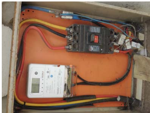
Figure 26. Main switch at Transformer
