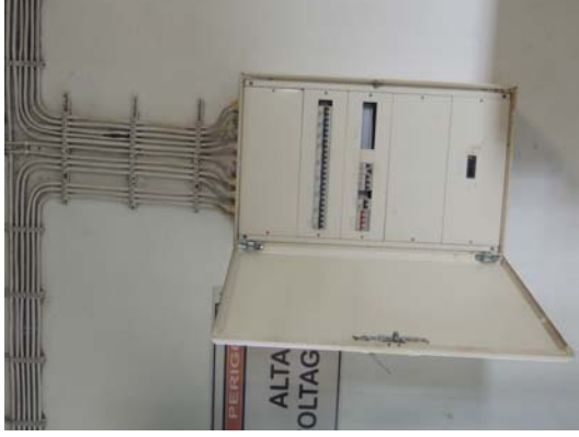
Figure 20. Control board of locksmith workshop
