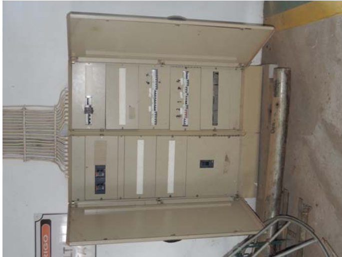
Figure 18. Main Distribution Board, in the Joinery workshop
