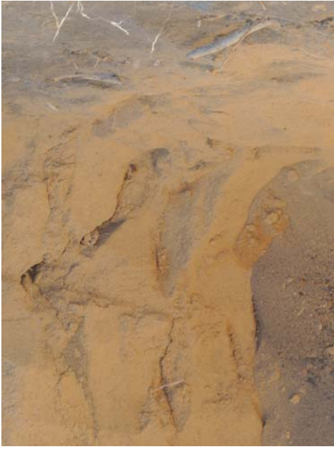
Figure 19. Detail of internal erosion
