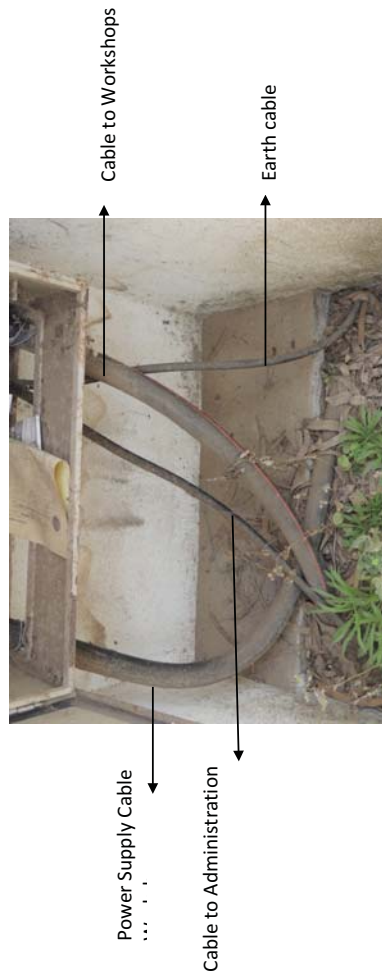
Figure 27. Cables at the Transformer
