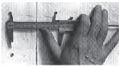
Figure 3.2.1 Crack Monitoring with Vernier Calliper on Concrete Wall (source: JET)
