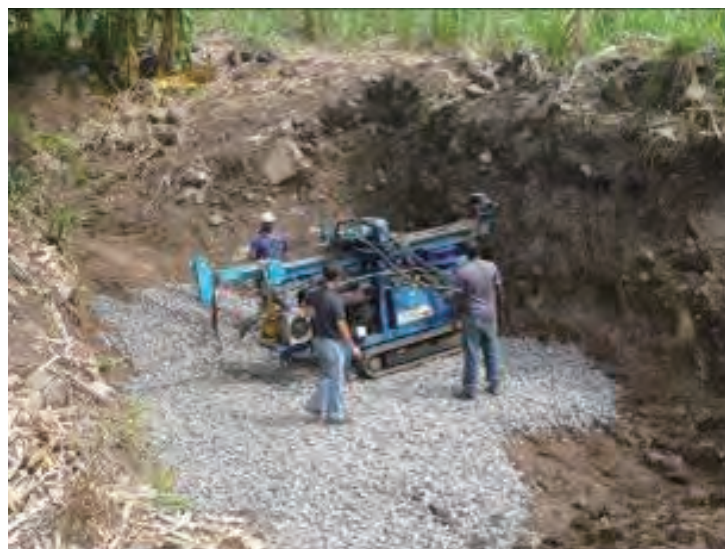
Photo A-3 Setting of drilling machine in the direction of the marked points (Source: JET)
