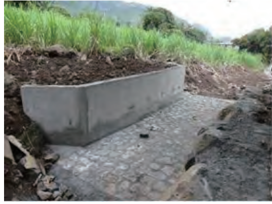
Photo A-5 Retaining wall for protection of mouth of drainage pipes and discharging channel (Source: JET)
