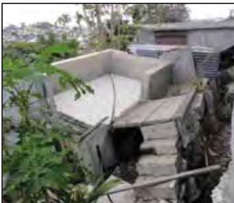
Landslide Damage (Vallée Pitot)
