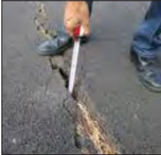
Crack on the Road
