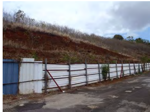
The existing retaining wall which collapsed was already removed, 2016
