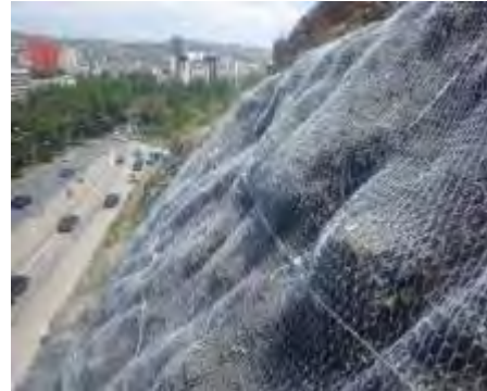
Photo 13 Real instance of a rockfall net (Source: JET)
