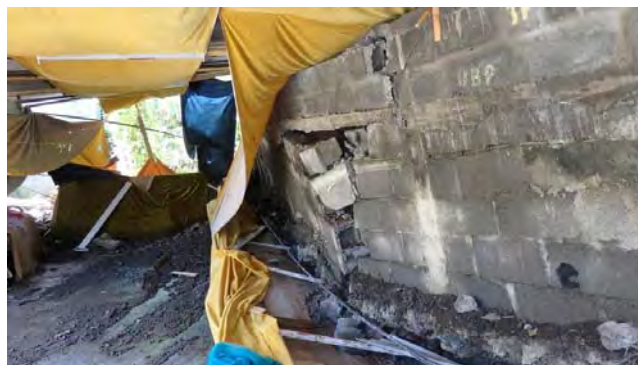
Photo 26 Failure of earth-filled road (Source: JET)
