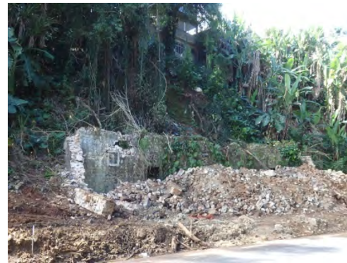
Photo 2 The slope in which a retaining wall (1.5 m high) is to be applied (Source: JET)
