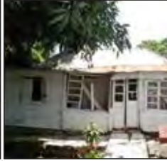
Deformation of the House
