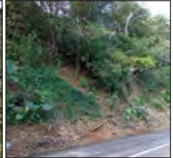
Slope covered by loose Soil is prone to Slope Failure
