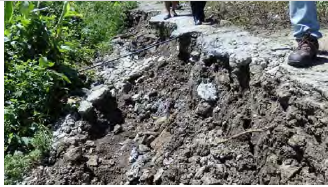
Photo 27 Failure of the concrete retaining wall of the mosque located down the slope (Source: JET)
