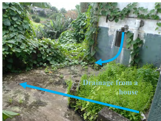
Photo 22 Domestic wastewater drainage, a likely cause of scarp erosion (Source: JET)
