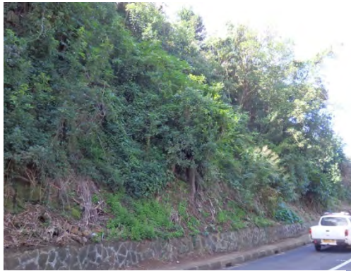
Photo 1 The slope near the end of the road is to be mortar-sprayed (Source: JET)
