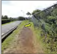
Fence Damaged by Slope Failure
