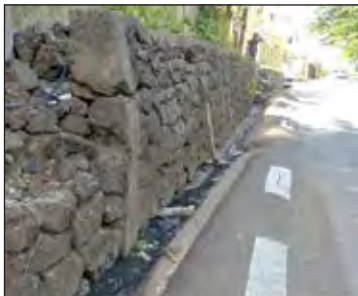
Landslide Damage (Quatre Soeurs)
