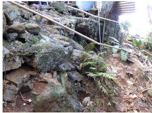
Photo 29 Part of the concrete below the foundation was scraped (Source: JET)
