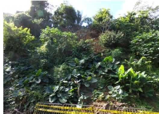
Photo 4 The upper part of the slope is to be mortar-sprayed (Source: JET)
