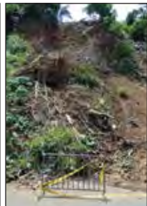
Slope Failure (Batelage)
