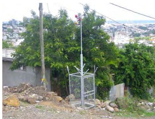
Figure 2 EWS in Vallée Pitot (Source: JET)
