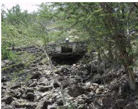
Photo 6 An example of a damaged drainage (Source: JET)
