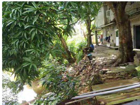
Photo 23 Current condition of the slope failure site (Source: JET)
