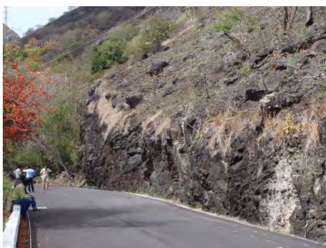
Photo 8 Planned location for a rockfall protection net on the side of the mountain (Source: JET)
