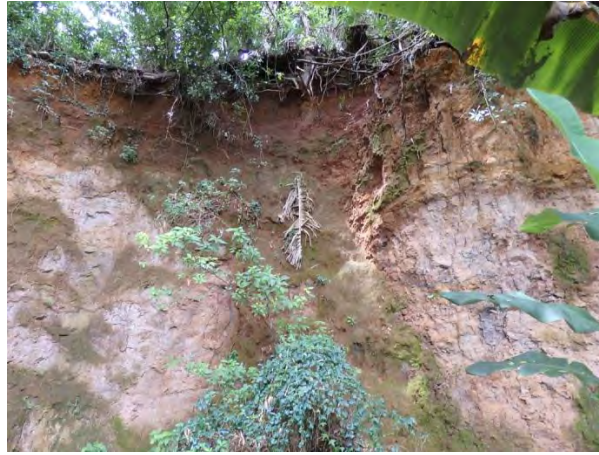
Photo 25 Cut-earth slope failure (Source: JET)
