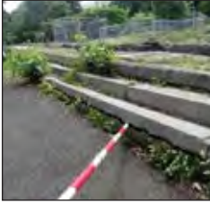
Deformation in the Steps
