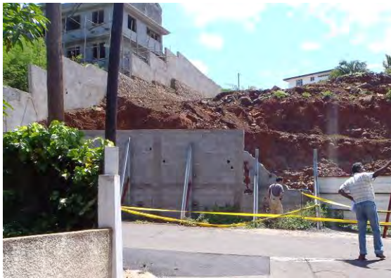
Existing retaining wall after the collapse, 2012
