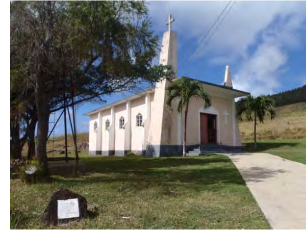
Excising Building (Church) No damage by landslide is found on this land, on the existing building (church).
