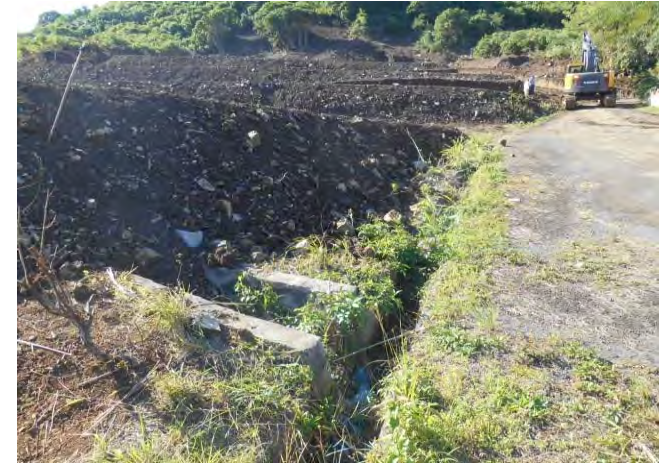
Photo-3 Lower part of the development area. Drainage of the road and slope are buried by debris.
