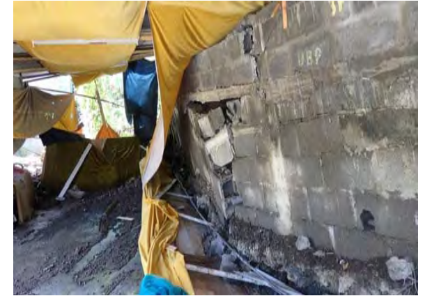
Photo-3 Damage of the concrete block wall of the mosque. The wall was inclined by lack of strength. The base of the wall was pushed up.
