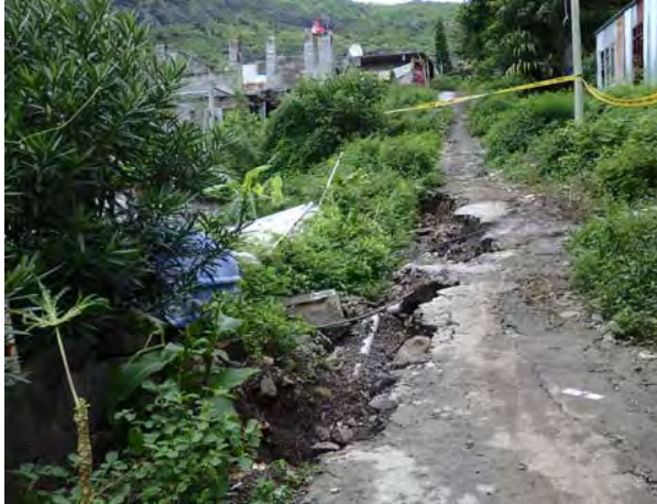
Photo-1 Full view. Long term rain water infiltrated through the road surface and the earth fill was saturated. The flash flood did not flow into the damaged part. That indicates after flash flood, the wall and road were collapsed. No leakage was observed from the sewage pipe.
