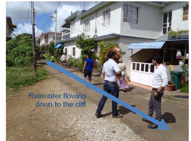
Rainwater flowing down the cliff from the road accelerates erosion of the cliff.
