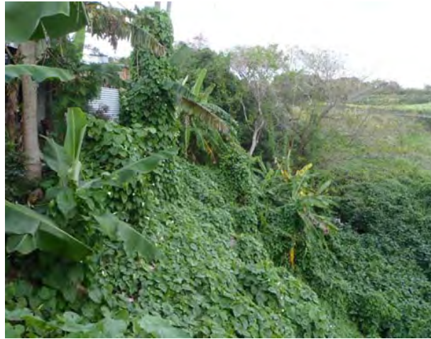
Unstable river bank slope behind a house
