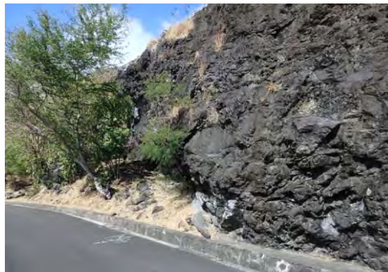
Photo-5 Cut slope with overhang. Middle part of the cut slope is cracky basalt. That part has been eroded selectively, and consequently, slope become over hang. The slope is planed to protect by fixing concrete.
