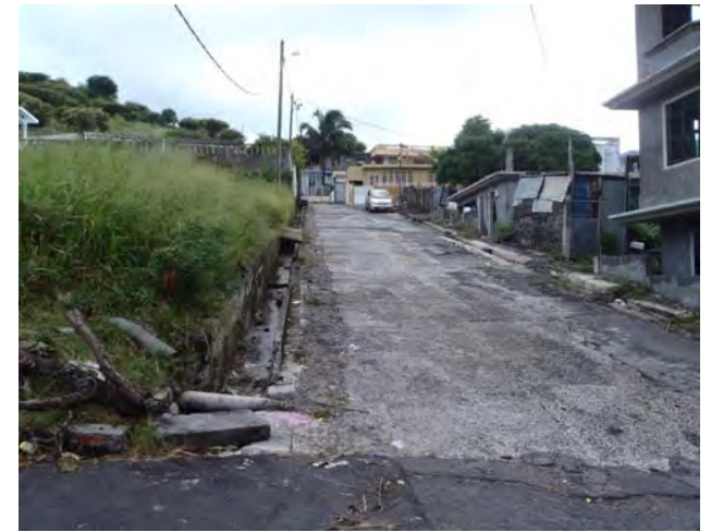
Existing Drainage of Road Side No damage by landslide is found on the existing open drains.
