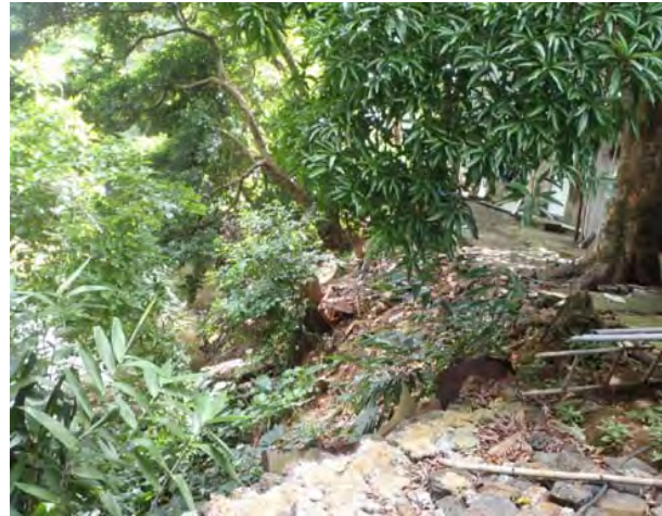
Unstable river bank slope behind a house
