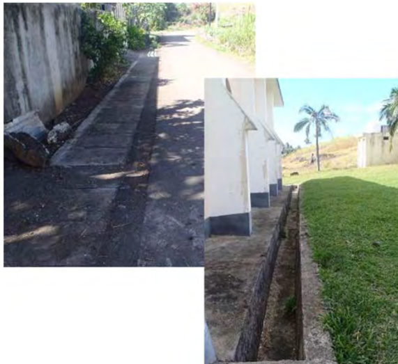
Existing Drainage of Road Side & Around Church No damage by landslide is found on the existing open drains.
