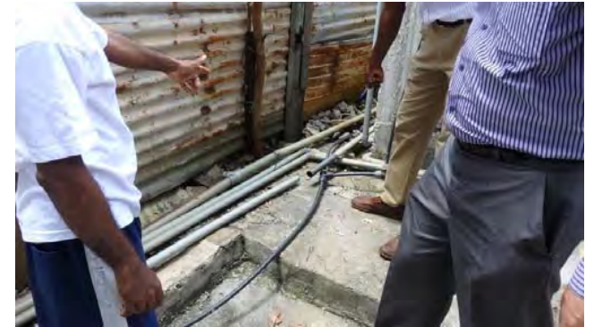
Photo-3 One another cause of the landslide is improper water treatment from the houses on the top of the slope.
