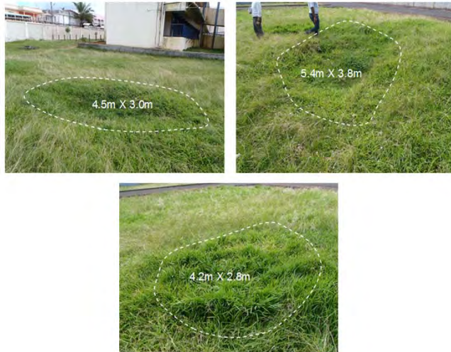
Current condition of three depressions in the green area
