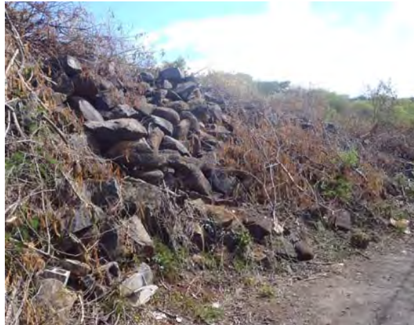
Unstable big boulders at toe of the slope
