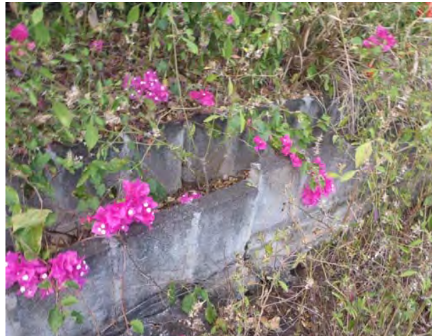
Excising Drainage The existing drainage need to be repaired.
