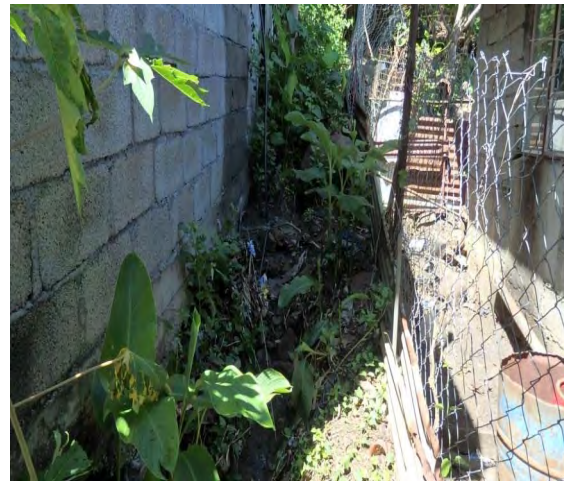
Photo-5 Some houses stand on the edge of the slope. Trace of flash flood on the floor of the mosque. Drainage water system is not well developed in surrounding area.
