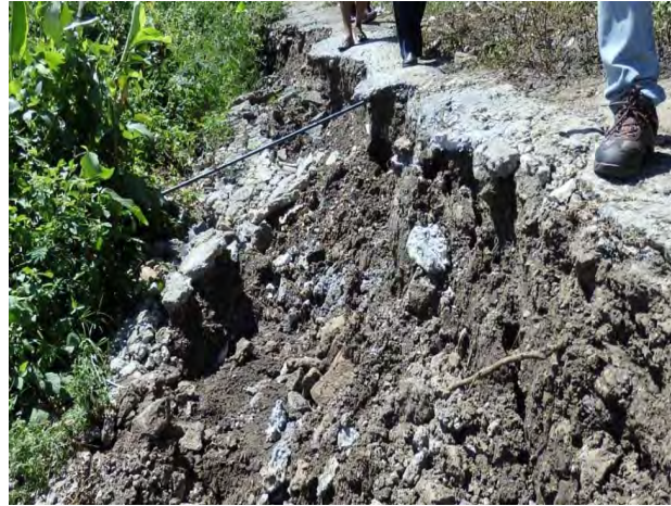
Photo-2 17m long, 3m wide and 0.5m deep collapse of the road
