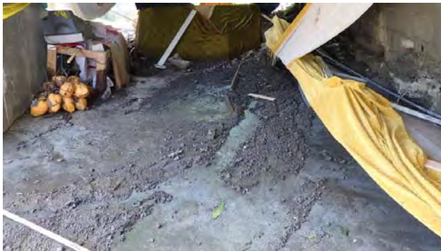
Photo-4 Trace of flash flood on the floor of the mosque. Drainage water system is not well developed in surrounding area.
