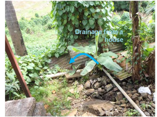
Drainage from a house accelerates erosion of the cliff
