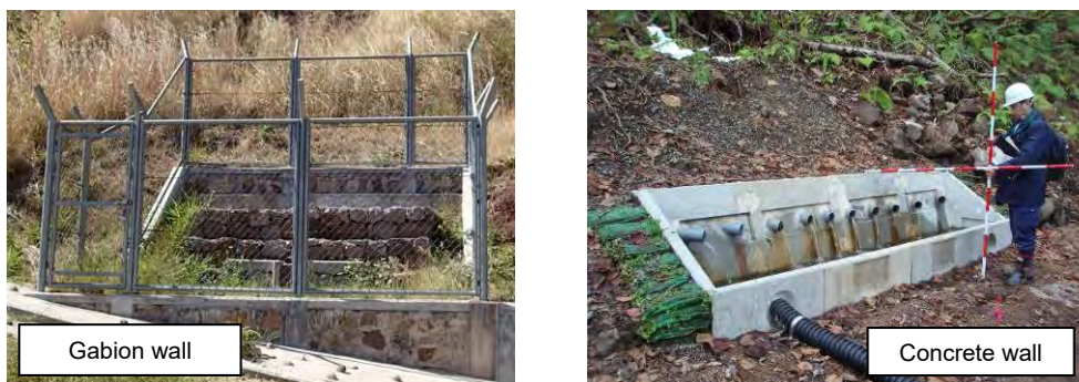
Figure 3.1.2 Example of retaining walls for outlets of horizontal drainage systems (Source: JET)
