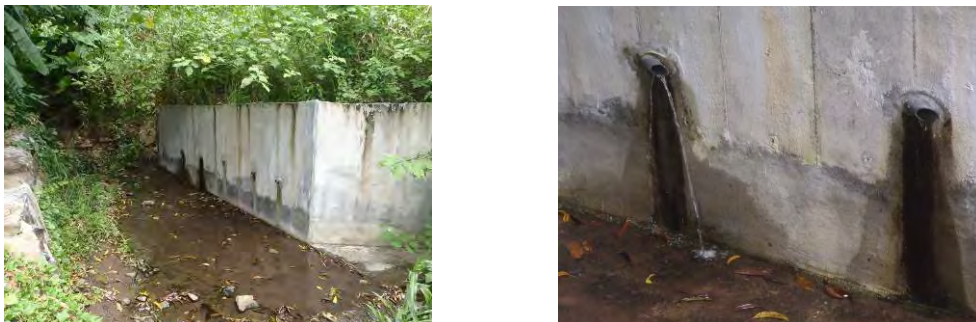
Figure 3.1.1 Horizontal drainage system in Chitrakoot, Block A (Source: JET)
