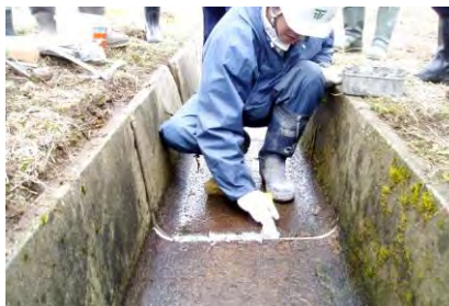
Figure 2.4.1 Example of repairing of crack on the surface drainage system (Source: JET)
