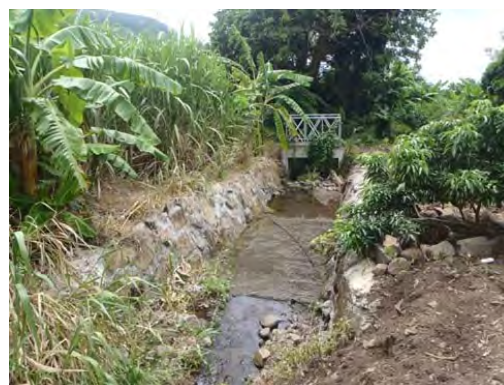
Photo 4 View of landslide countermeasure, upgrade drainage, UD-2, 08 th March 2016 (Source: JET)
