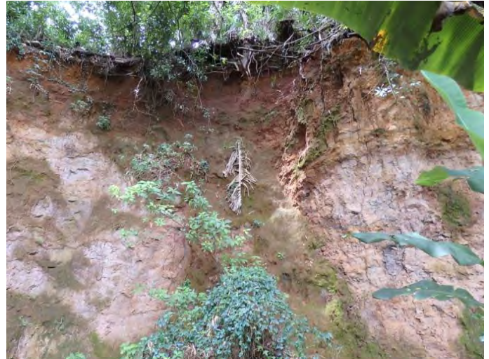
Cut slope failure, Pilot Bel Air
