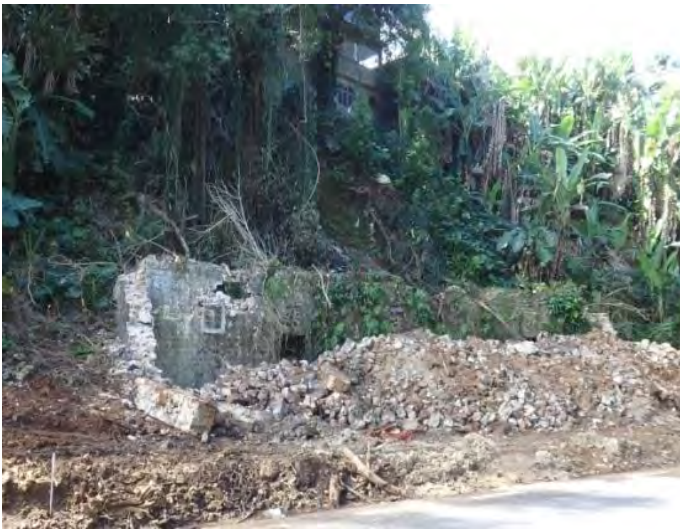
The slope in which a retaining wall (1.5 m high) is to be applied, Batelage
