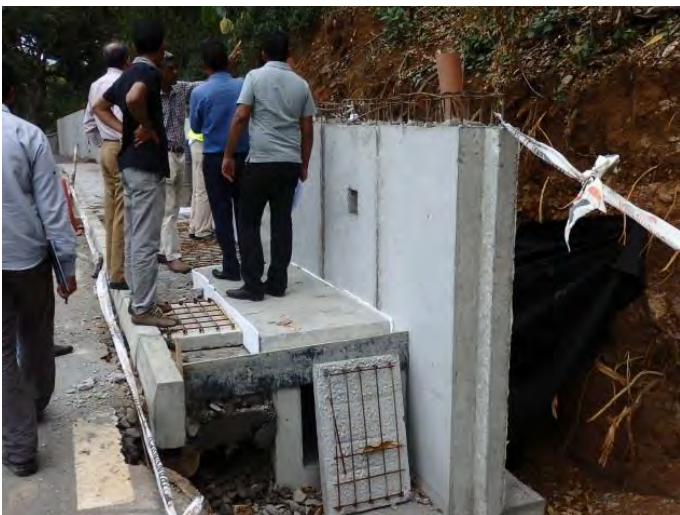
Construction of retaining wall at a place of possible slope failures, Batelage
