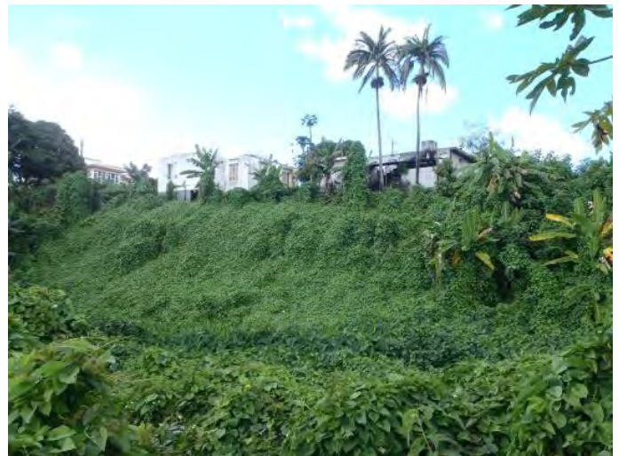
The investigation spot where two houses sit near the scarp, Camp Garreau, Flacq
