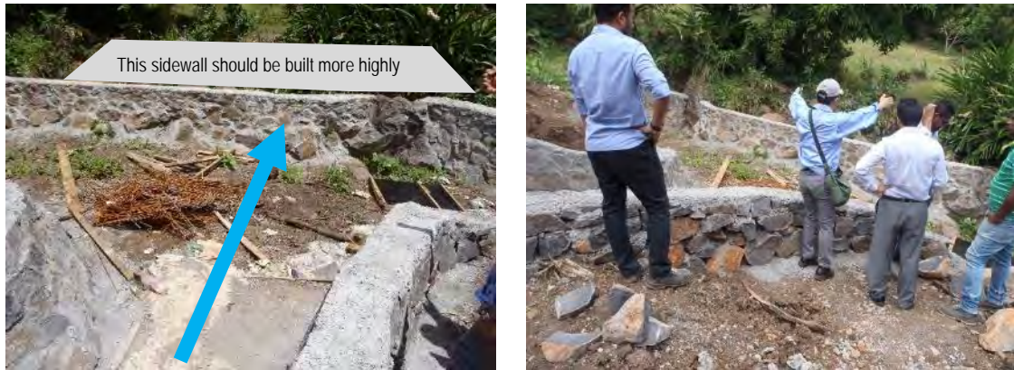
Figure 2 Bend (near BR-6) of New Channel, NCH1, needing building up (Source: JET)
