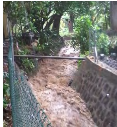
Photo 4 End part of the Reinforced Upgrade Drainage, RUD-1, during the rainy season in January 2015 (Source: JET)
