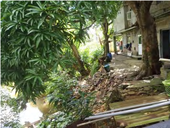
Current condition of the site with slope failure and river erosion, Kewal Nagar Belle Rive
