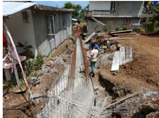
A.2: Drain (Source: JET)
