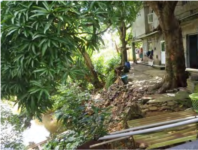
Current condition of the site with slope failure and river erosion, Kewal Nagar Belle Rive
