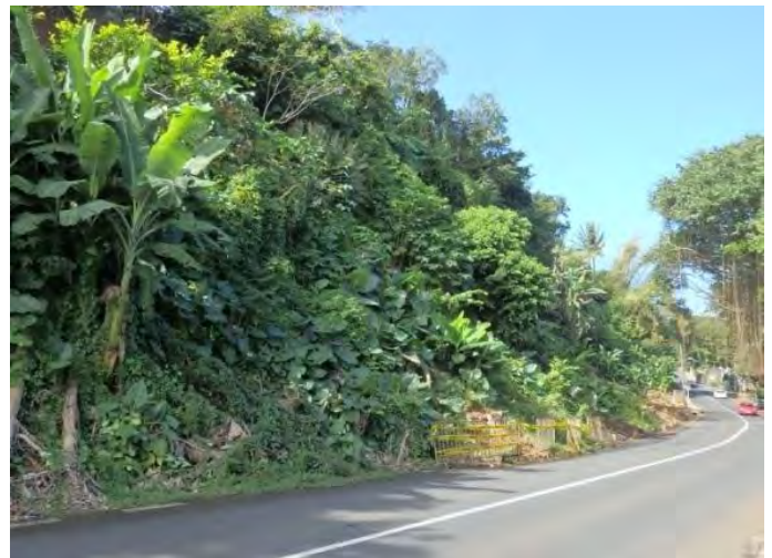
The slope at middle of the road in which a crib wall is to be applied, Batelage
