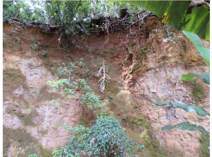
Cut slope failure, Pilot Bel Air
