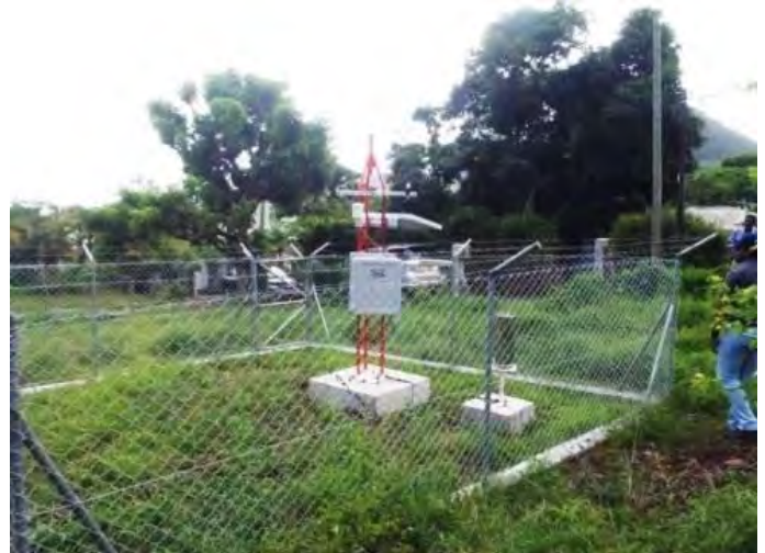
Automatic Weather Station (AWS) for early warning installed by the Mauritius Meteorological Services (MMS), Chitrakoot
