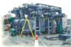
Black Point 420kV GIS CLP Power (Hong Kong)
