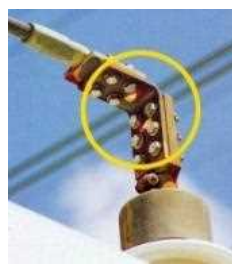
Overhead line termination
