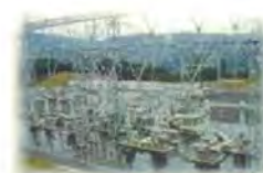
Chizu 550kV GIS Chugoku Electric Power co. (Japan)
