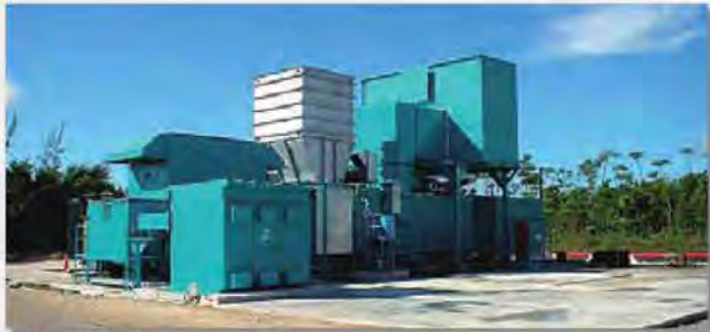
H-25 Gas Turbine Project (Bahamas)
