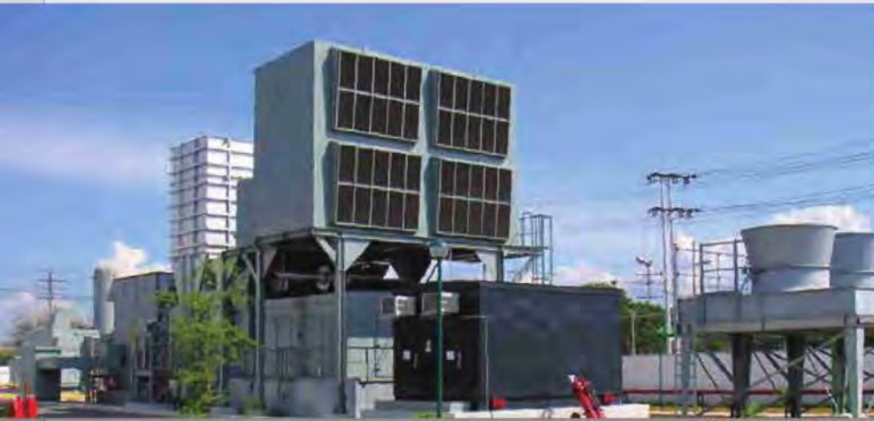
H-25 Gas Turbine Project (Venezuela)
