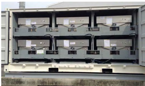
6 NAS Modules inside
