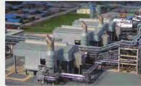
H-25 Gas Turbine Project (Indonesia)
