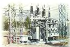
The first GIS in Japan Himeji 84kV GIS Kansai Electric Power co. (Japan)
