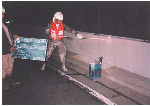
Photo 5.2.9.8 coating លើគេ
