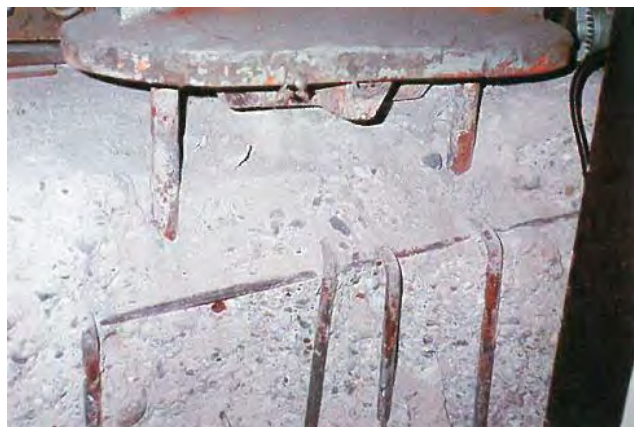
Photo 5.2.4.3 ខូចខាតបេតុង chipped off
