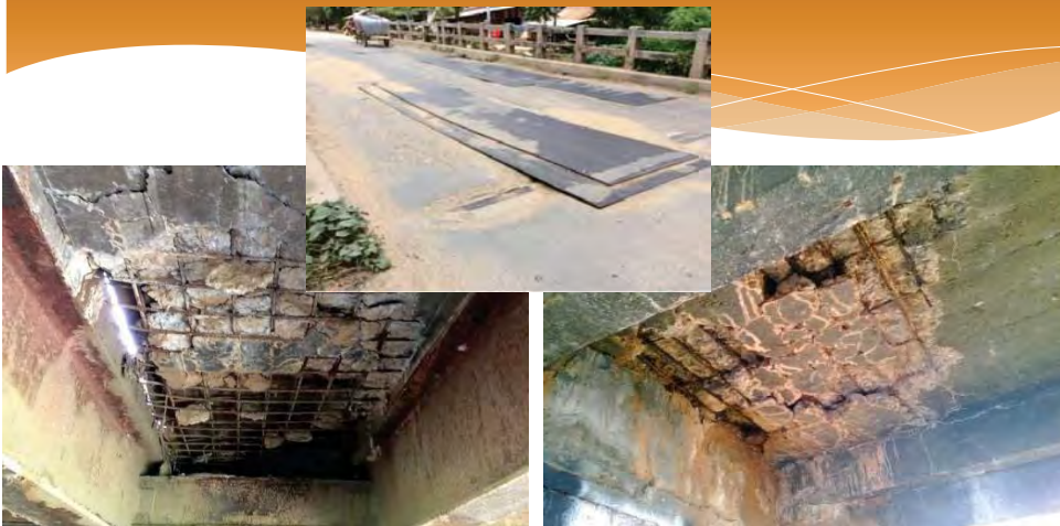
Serious structural defect on concrete slab deck
