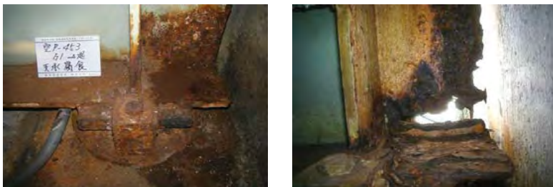
Corrosion of end of girder (In Japan)
