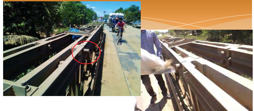
Damage of Bailey bridge (Loosing of a pin)
