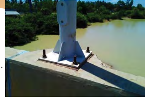
Lighting pole (Fixed by only 4 anchors)
