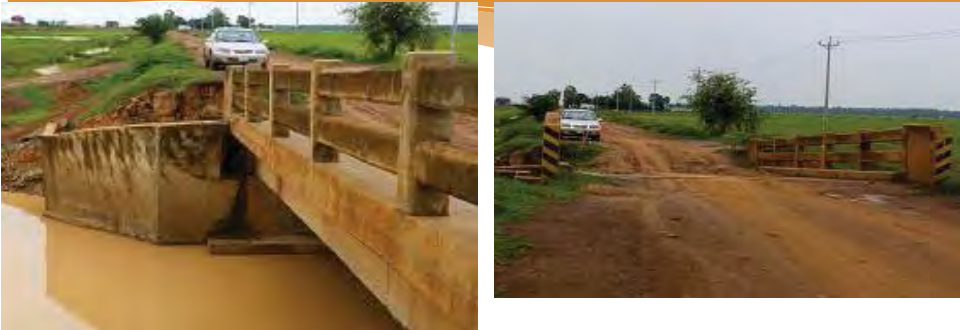
Abutment or pier unstable by scouring (Settled due to back filled soil washed out by scouring)
