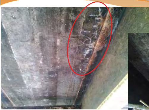
Phase 4 condition (Alligator crack)
