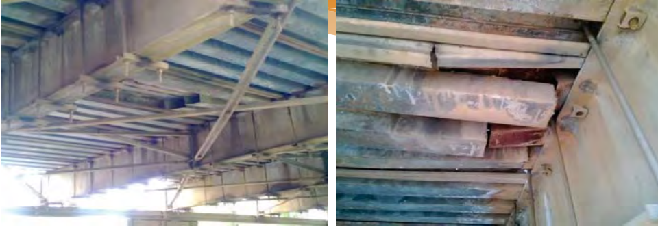
Serious structural defect on steel slab deck (Fatigue crack)
