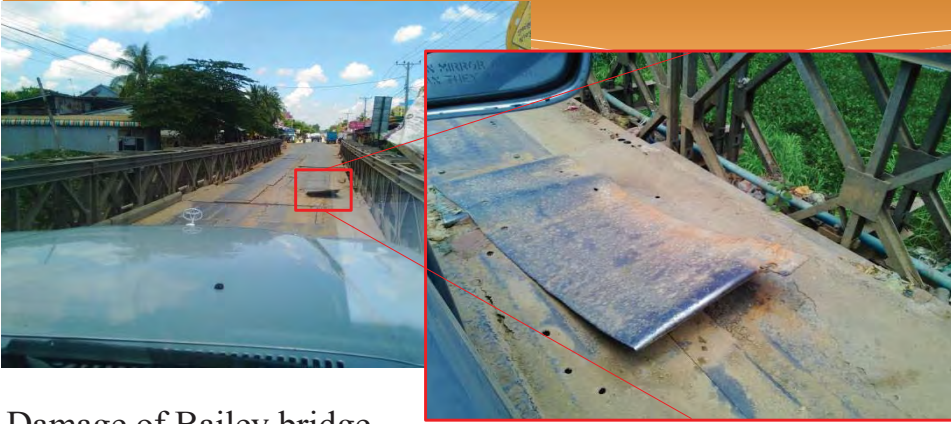
Damage of Bailey bridge ( Detachment of reinforced steel plate due to loss of bolt connection.)
