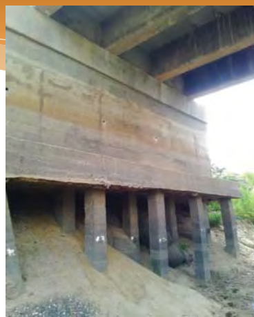
Scouring and broken pile (RN14)
