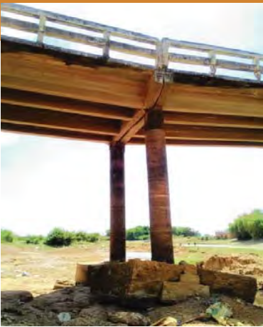
Scouring and settle pier(RN8) (This bridge is out of service)
