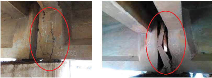
Crack at the end of concrete girder (Chroy Changva bridge)
