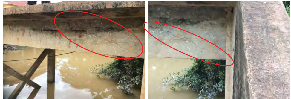
Crack at the end of concrete girder (PN265E bridge)
