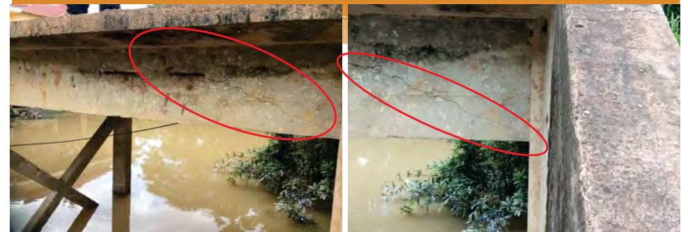
Serious structural defect on concrete girder (Shear crack)
