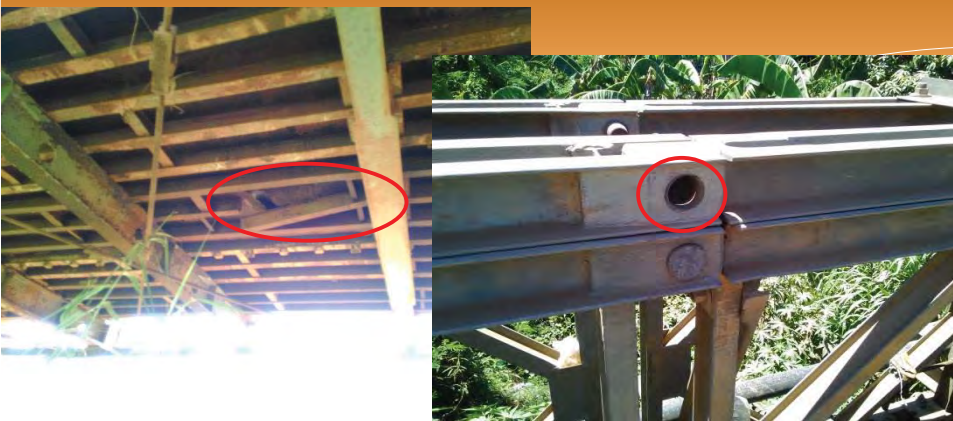
Damage of Bailey bridge (Left : Broken rib Right : Loss of a pin)
