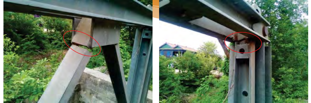
Serious structural defect on main girder or truss girder (Fatigue crack)
