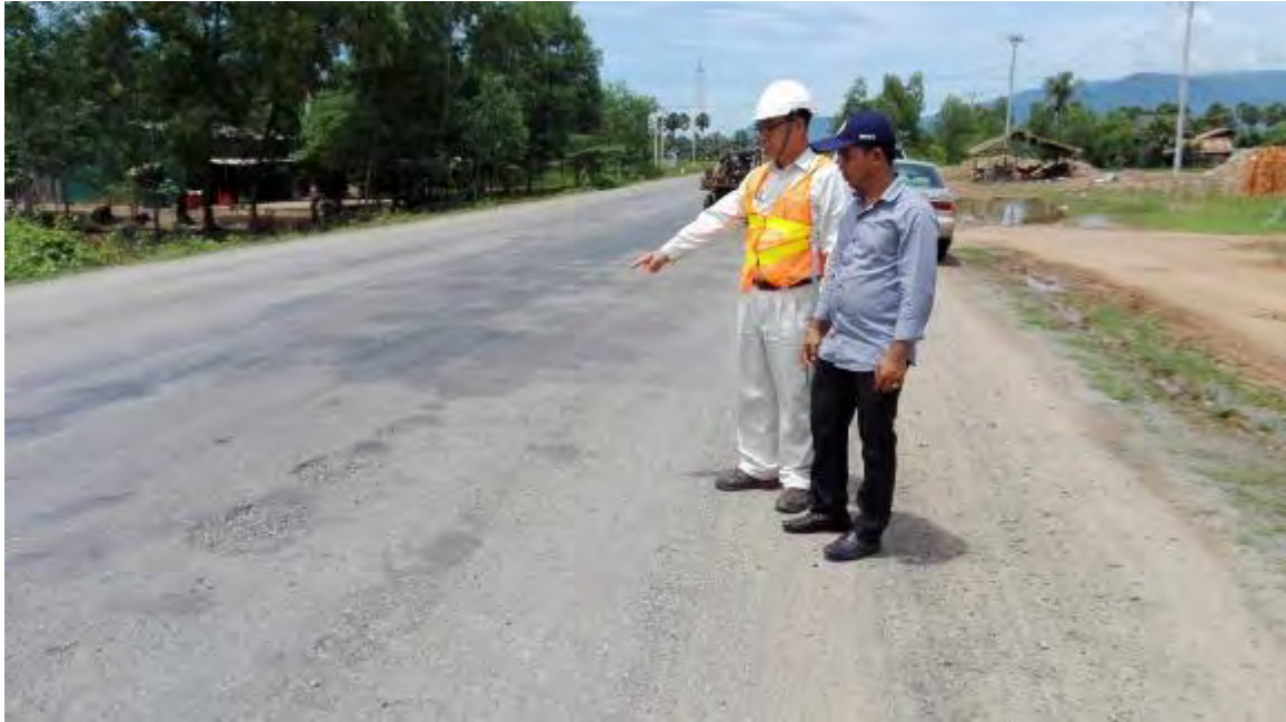
Photo 7-1 Observation of Road Maintenance Works by DPWT in Kampot Province (NR3 PK138~140km Problem Area)
