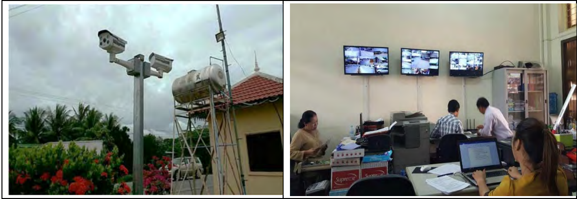
Figure 9-55 Picture of Surveillance Camera System
