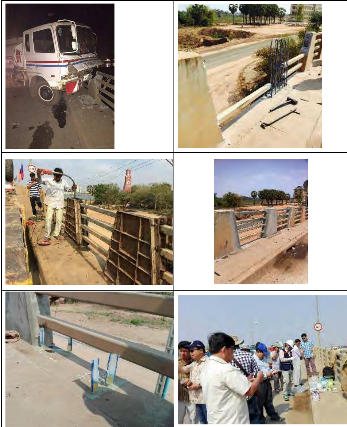
Photo 7-22 Repair of the Damage at Kizuna Bridge and Demonstration of Crack Sealing Method
