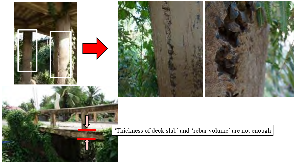
Photo 7-5 Insufficient strength capacity
