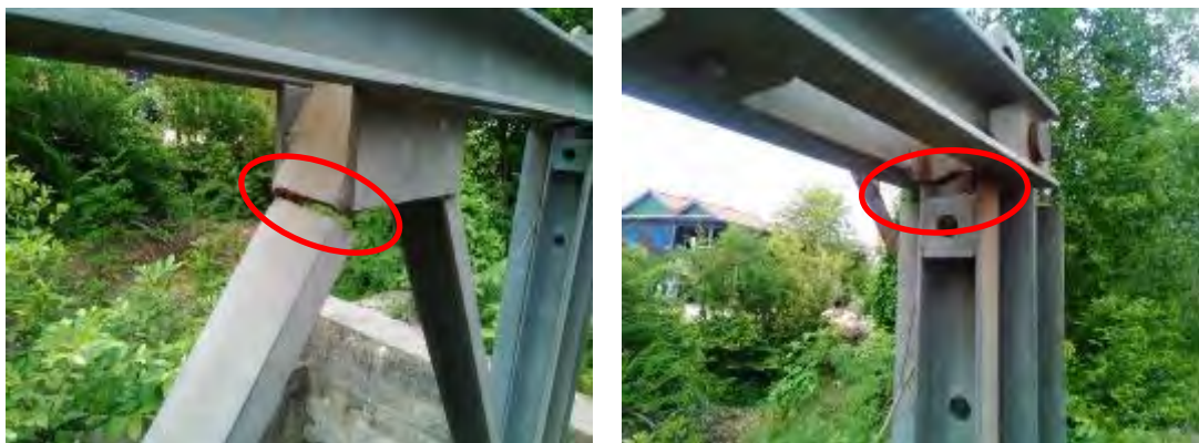
(E) Serious structural defect on main girder or truss girder (Fatigue crack)
