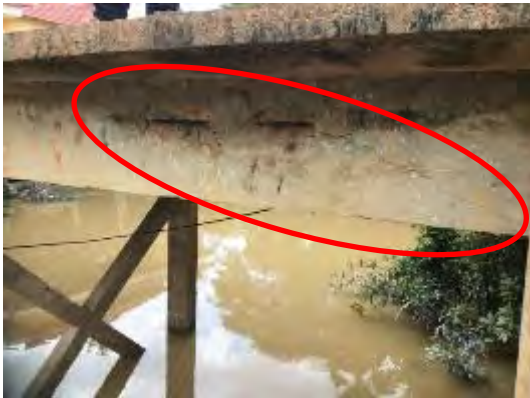
Shearing crack on concrete girder
