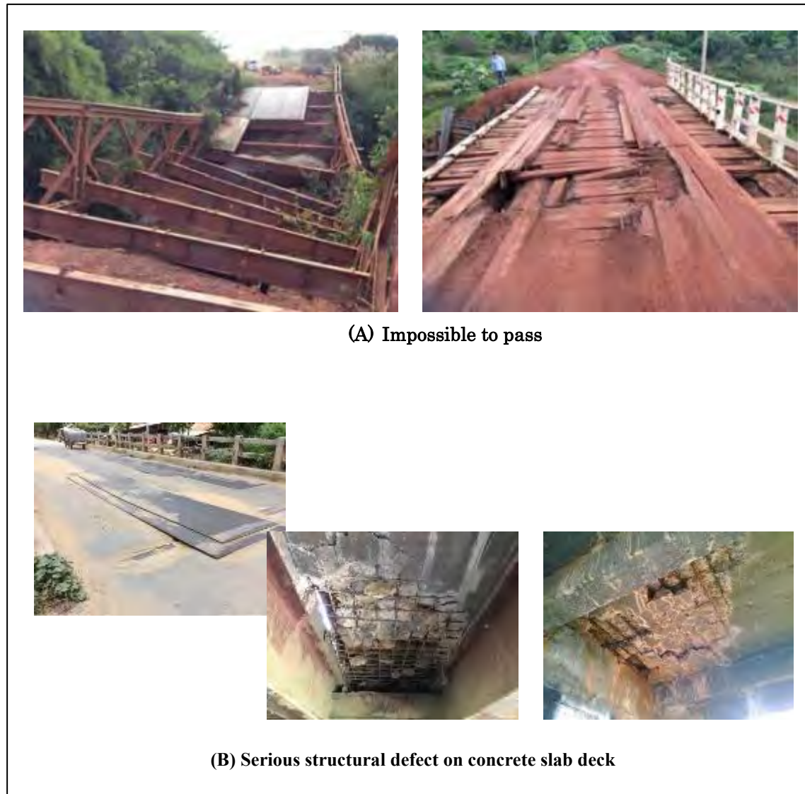
Fig.1 Sample Photo of a Seriously Damaged Bridge (1)
