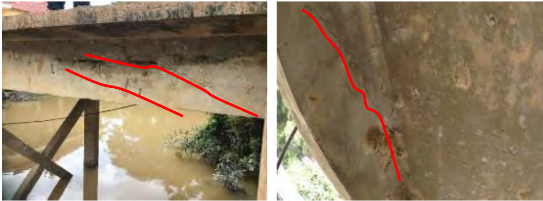
(C) Serious structural defect on concrete girder (Shearing crack)
