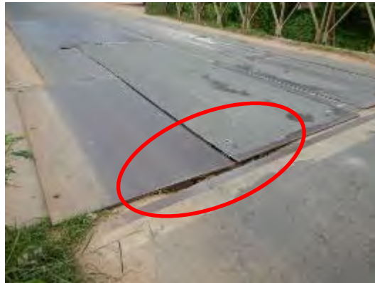
Fatigue crack and hole on steel deck
