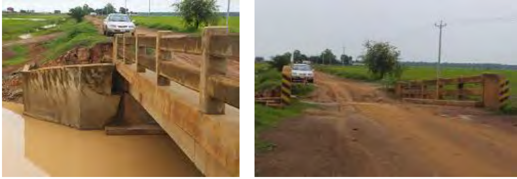
(F) Abutment or pier unstable by scouring (Settled due to back filled soil washed out by scouring)
