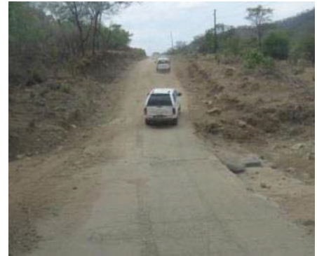
Access road to local health center submerging in rainy season (Southern Province)
