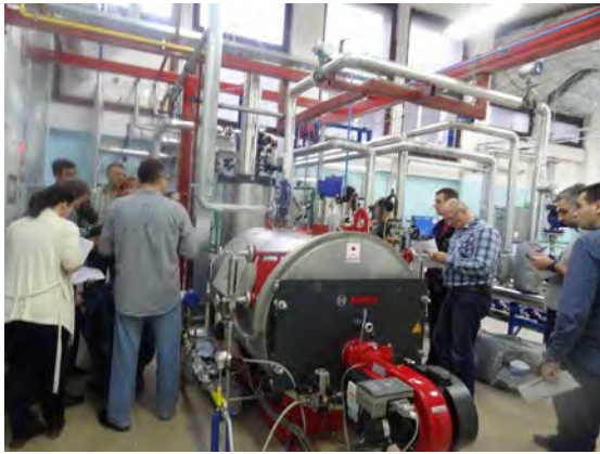
Practical Training for Boiler
