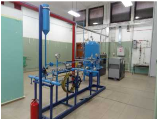
Air Compressor Unit
