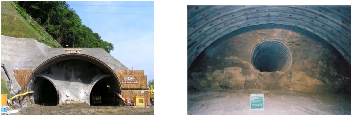
Figure 3-24 Side Drift Advancing Method (left) and Top Drift Advancing Method (right) (Source: JICA project)
