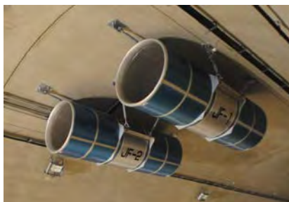
Figure 6.2 Ventilation Equipment (free-suspended Jet Fan)
