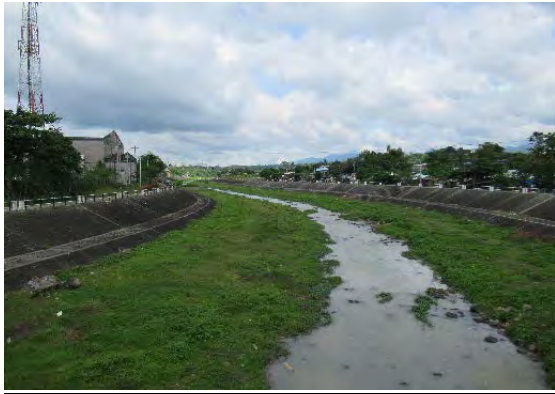
Improved Anilao River (upstream view) Photo: JICA Project Team F1: Flood Control in Ormoc City, Philippines
