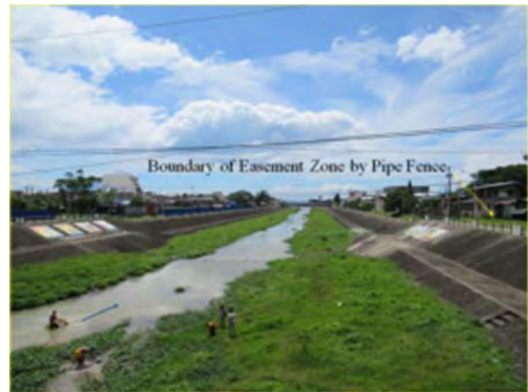
River Improvement in the Mid-stream to Downstream Reaches of the Anilao River
