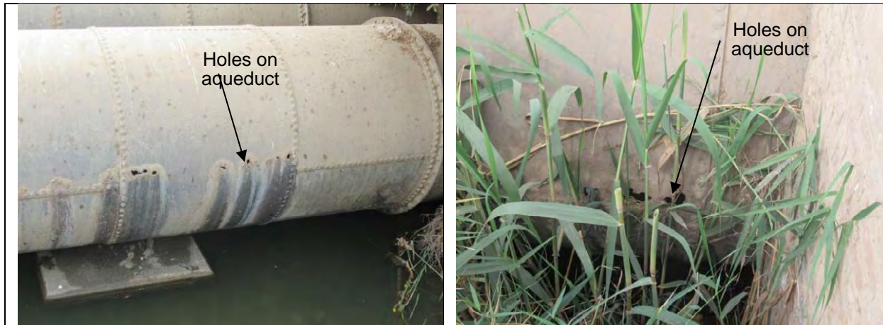
All of the 4 aqueduct has holes that leaks the scarce water resource into drain
