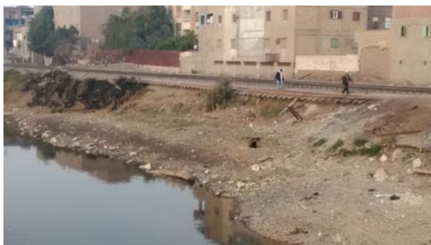
Destroyed railway line along the bank of the canal
