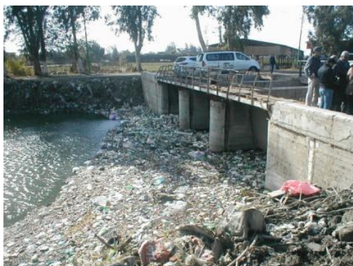
Accumulated garbage in upstream of Mehala Menouf Regulator
