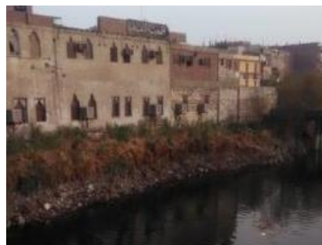
Progressive erosion on the foundation of the house
