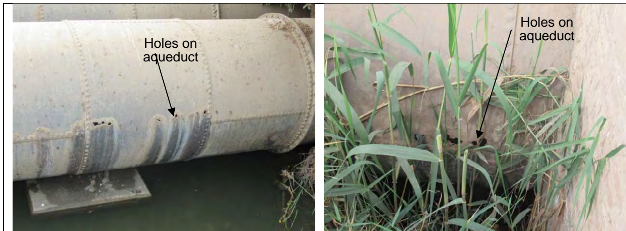
All of the 4 aqueduct has holes that leaks the scarce water resource into drain
