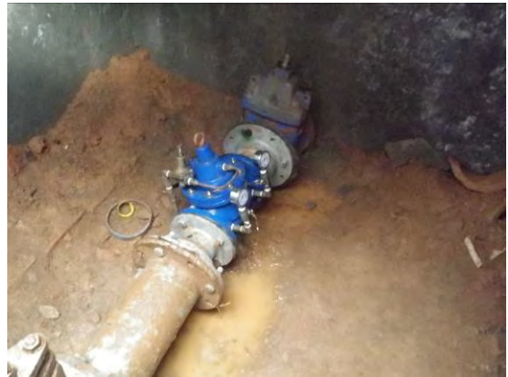
Pressure Reduce Valve Lilongwe North Zone (Jul.31, 2017)
