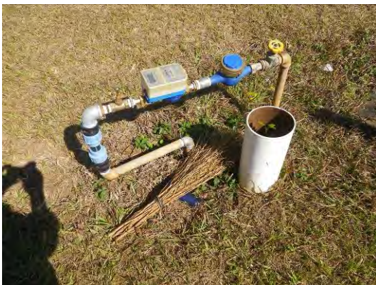
Prepaid Water Meter LWB HQ (Jul.22, 2017)
