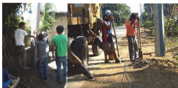
Manual Digging for Poles Since there is No Boom Truck with Digger.
