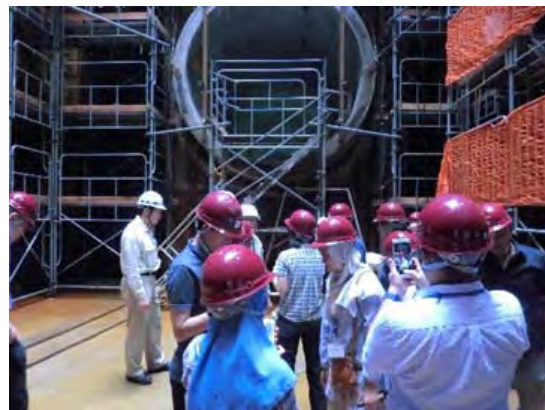
Site Visit at Construction site of Drain laying by Shield Method (1 September, 2016)
