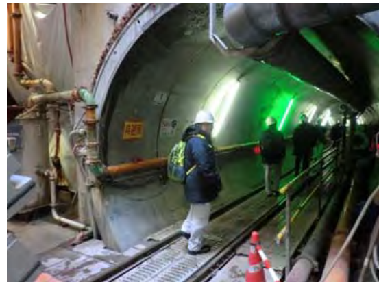
Site Visit at Construction site of Drain laying by Shield Method (25 February, 2016)
