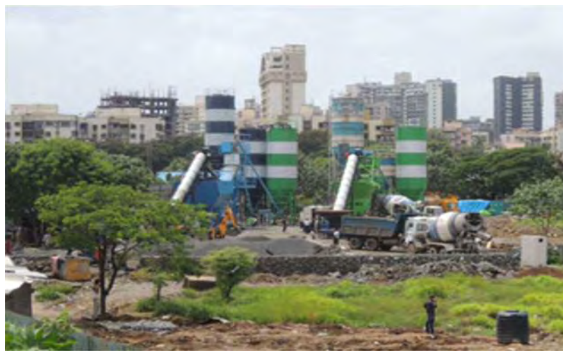
Figure 8.1.5-5 Fresh Concrete Plant
