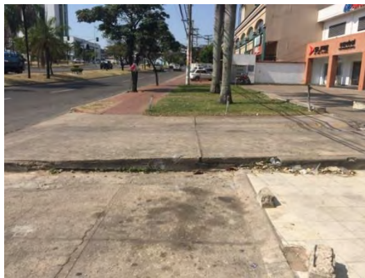
Source: JICA Study Team Figure 2.6-12 Pictures of sidewalk discontinuity
