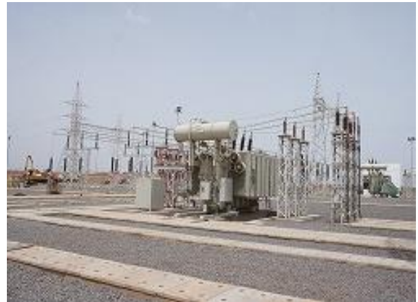
Jaban As Substation, Djibouti
