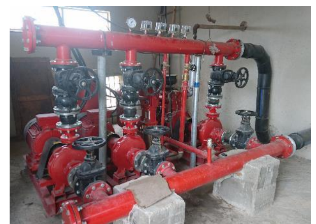
Hydrant System, Bole Lemi Industrial Park, Ethiopie
