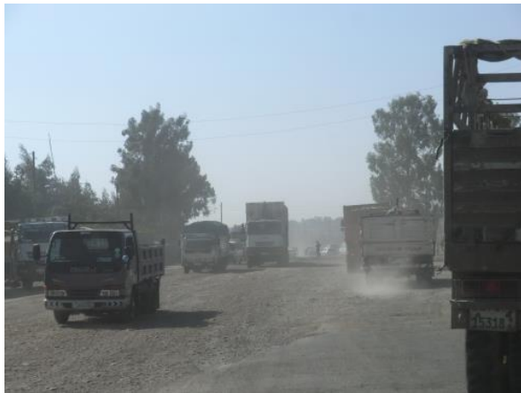
Deteriorated Road on the Djibouti Corridor (Ethiopia)
