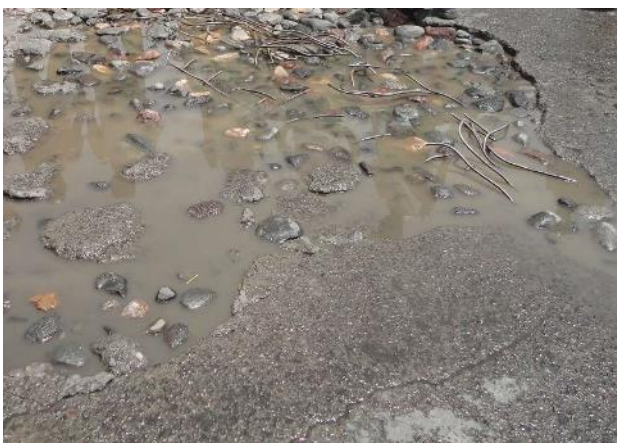
Damaged Road Surface of National Route 1, Djibouti
