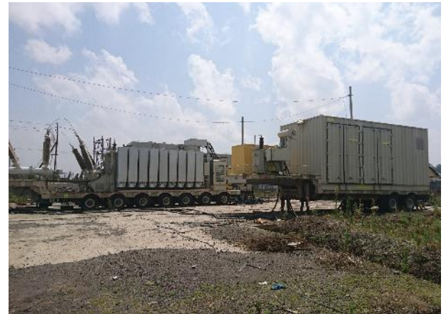
Power Station, Bole Lemi Industrial Park, Ethiopia
