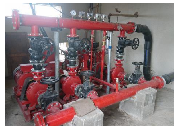
Hydrant System, Bole Lemi Industrial Park, Ethiopia
