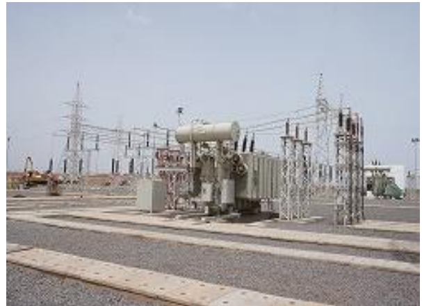
Jaban As Substation, Djibouti
