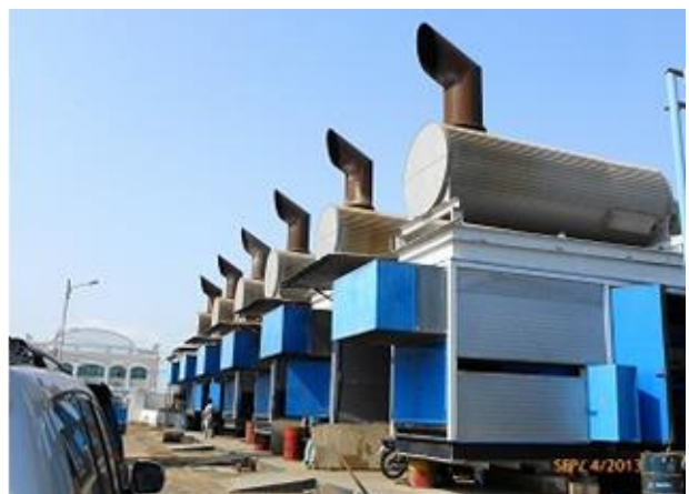
Marabout Power Station (fuel: Gas-oil), Djibouti
