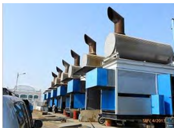
Marabout Power Station (fuel: Gas-oil), Djibouti
