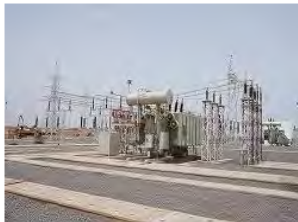
Jaban As Substation, Djibouti
