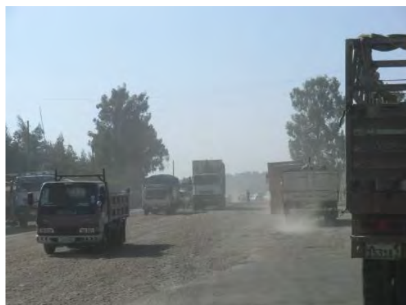
Deteriorated Road on the Djibouti Corridor (Ethiopia)
