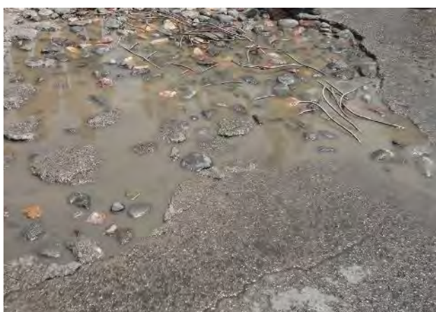
Damaged Road Surface of National Route 1, Djibouti
