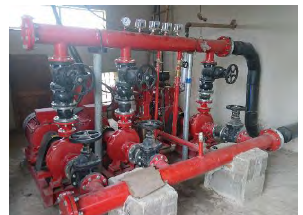
Hydrant System, Bole Lemi Industrial Park, Ethiopia
