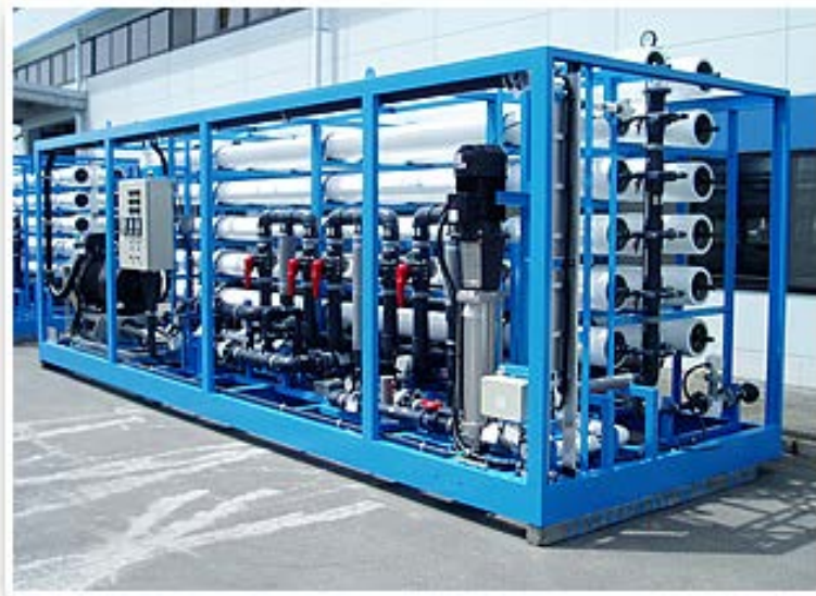
Picture 5-6 Desalination Device
