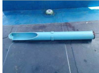
Water intake pipe
