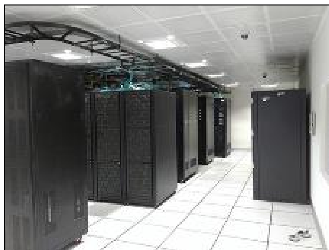
Figure 2-4 Server Room in KSDC
