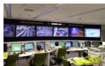
Central Monitoring System
