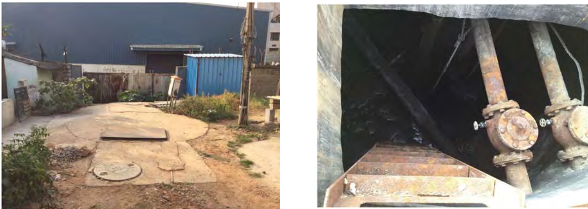
Photo 10.2.22 Manhole Type Pumping Station (presently not being operated)
