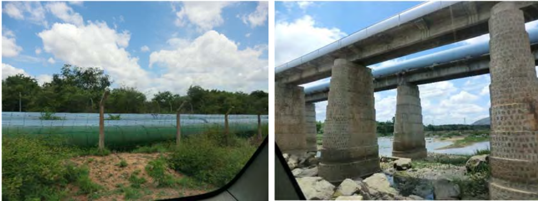
Photo 14.2.1 Conveyance Pipeline (1) Conveyance Pipeline crossing Shimsha River (2)
