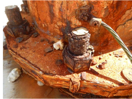
Decay of the basement of the antenna tower
