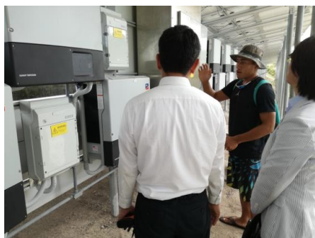
Field Explanation by the Engineer
