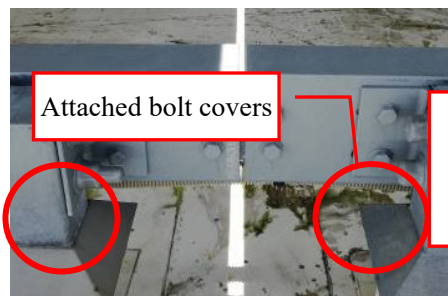
Covers on the Bolts in the Frame
