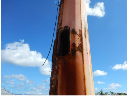
Decay of the antenna tower
