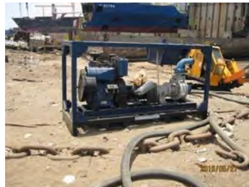
P.V-5 Mobile fire pump
