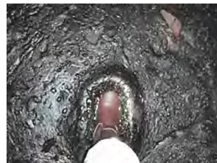
Sludge before cleaning
