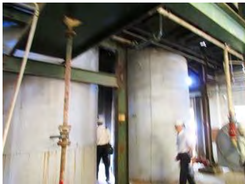
Capacity 7,000 KL / year Product Tank after 1 st distillation
