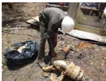
No gloves during glasswool removal (Normal yards)
