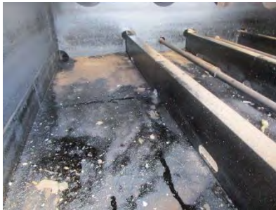
Oil still remaining inside fuel tank after cleaning (yard in process of verification)
