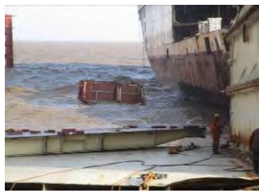
Blocks being dropped in the sea / in the inter-tidal zone (Normal yards)
