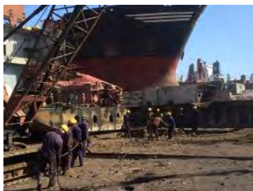
Blocks being dropped inside the ship not to the inter-tidal zone (NK certified yard)
