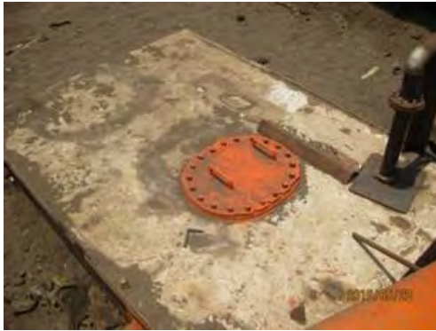
P.V-7 Dirty oily water tank(5,000 liter)
