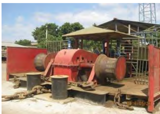
P.78 75 t Winch with fence
