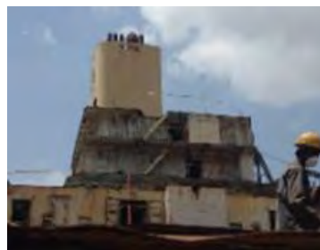
Warning tape to indicate the risk of working at height (NK certified yard)
