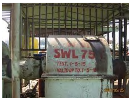
P.19 75 t Winch with fence
