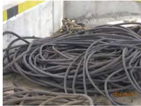
P.5 wire storage space is sunken in ground
