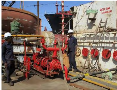
Fire fighting facility (Normal yards)
