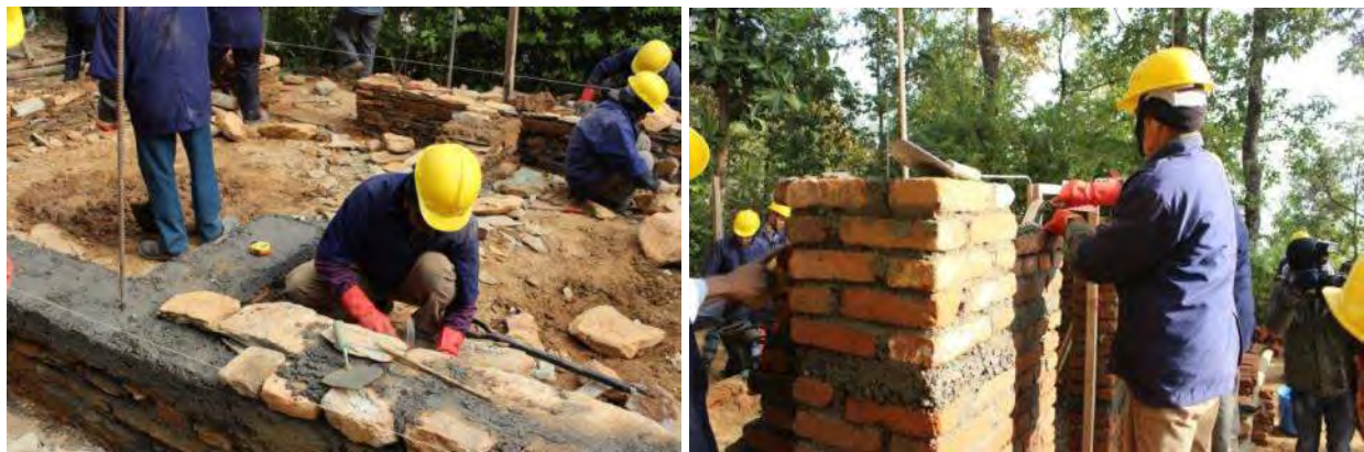
Source: JICA Project for the Transitional Project Implementation Support for Emergency Reconstruction Projects Picture 2.1 House Reconstruction Training for Masons
