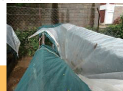
Collapsing shade due to heavy rains
